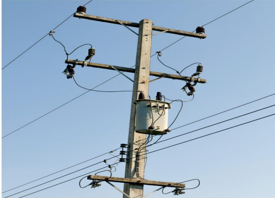
Figure 3.3: Utility Distribution Feeders
