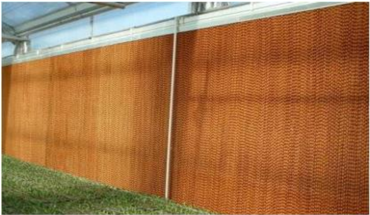
Figure 2.8 Fan and pad greenhouse evaporative cooling system [22]
