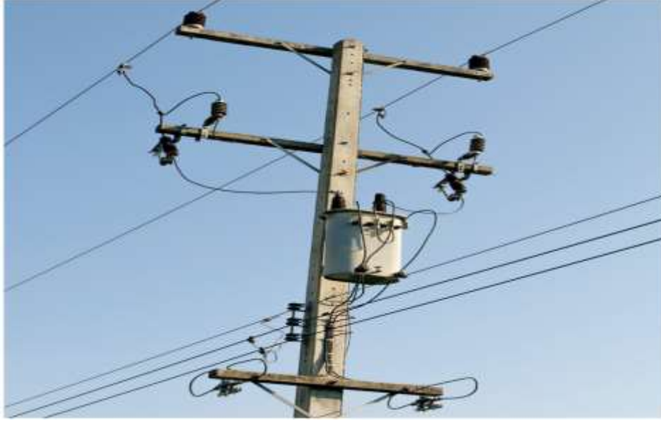
Figure 3.3: Utility Distribution Feeders
